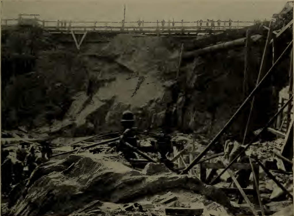
Looking east at Seventh Avenue. Approach to new Pennsylvania Terminal, with Cameron Pump removing 400 gallons drainage water per minute from the diggings to the sewer 65 feet above.
